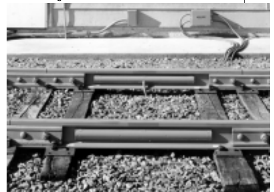
View of a Weighline installed
