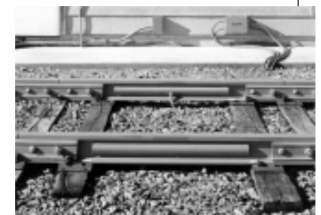
View of a Weighline installed
